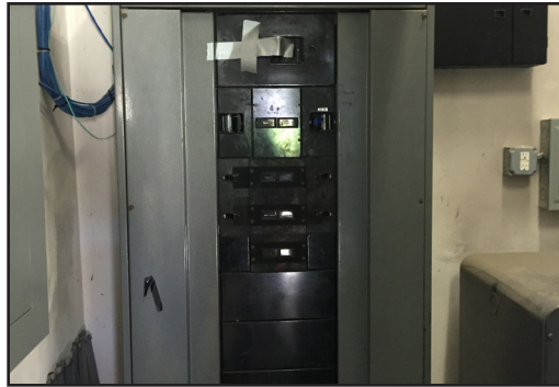
Main 800A 277/480V Switchboard
