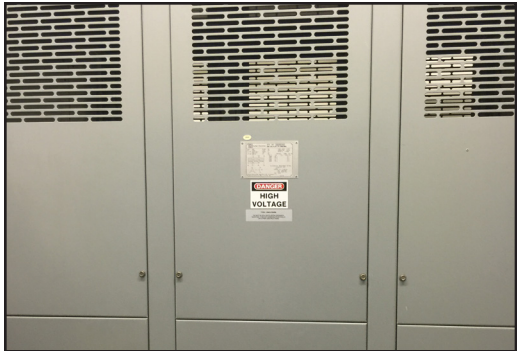
300kVA 4160-277/480V Dry-type Transformer
