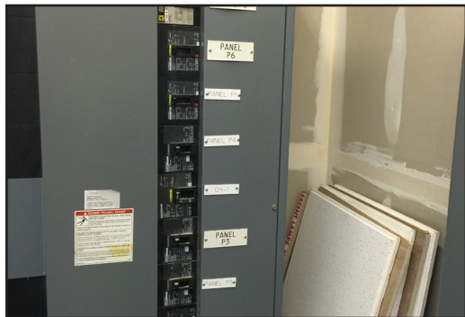
Main 2000A 120/208V Distribution Board
