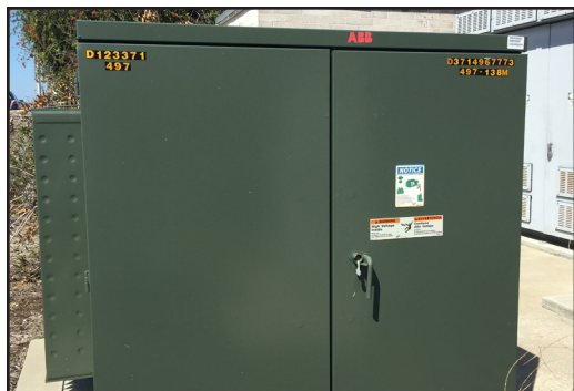
SDG&E Padmount Transformer
