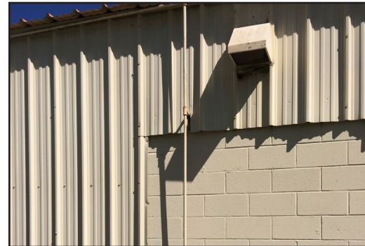
Building 4200 - Low pressure gas line running exposed along building exterior.
