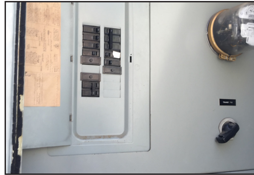
Main Distribution Board with Interior Panel Board
