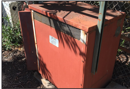
Abandoned Fire Pump Transformer
