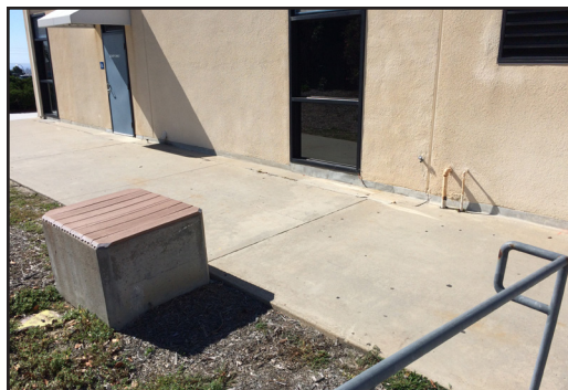
Building 3000 - Gas Pressure regulator inside concrete vault.
