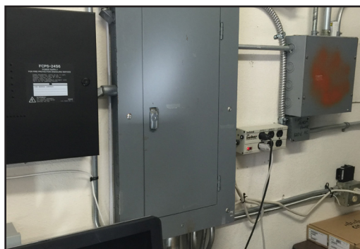
Building 100 - Panel boards Typical
