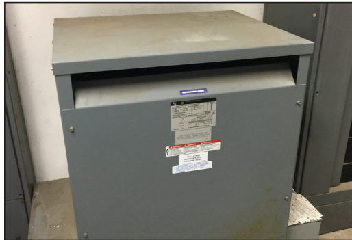
112.5kVA, 480-120/208V Transformer
