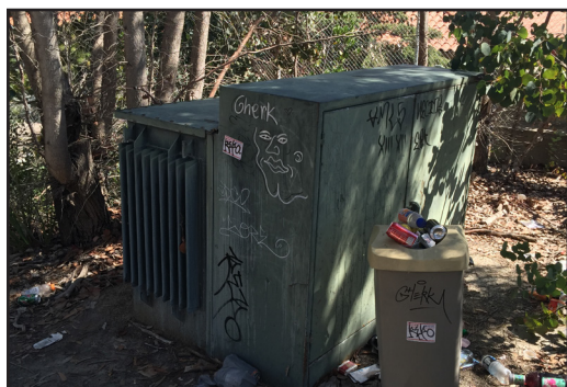
4.16kV-277/480V Padmount Transformer
