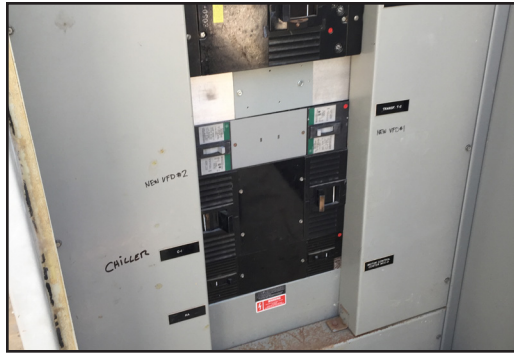
Main Distribution Board
