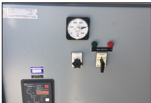
Main 5kV Breaker Cubicle and Protection
