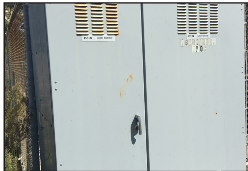
Main Distribution Board serving Fire Pump
