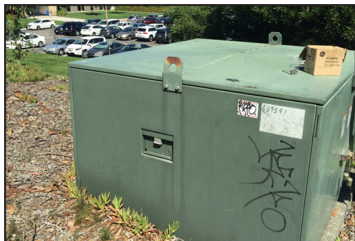
15kV Selector Switch
