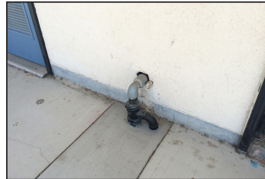
Building 3500 - Low pressure gas into building.
