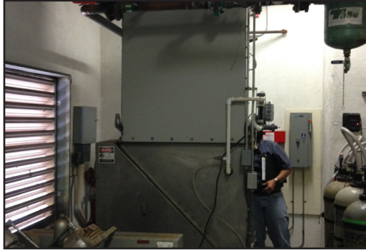
Typical Water Source Heat Pump Closed Circuit Cooler
