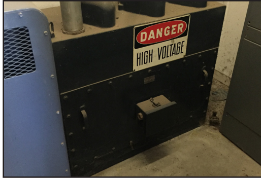
5kV Oil Fused Cutout
