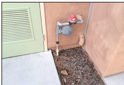
Building 900 - Gas supply into building with gas pressure regulator along building exterior.
