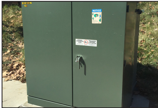
Typical SDG&E pad mount transformer
