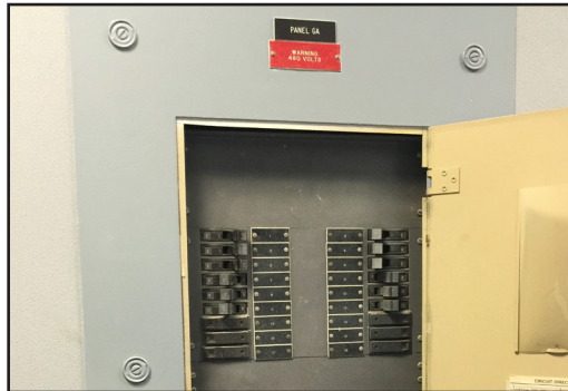
Main 120/208V Panel Board
