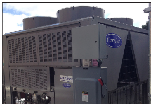
Building 1000 - Air-cooled chiller
