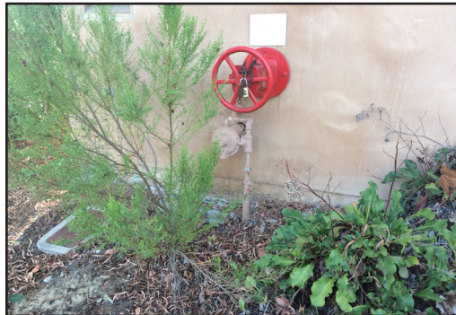
Building 700 - Gas supply into building with gas pressure regulator along building exterior.
