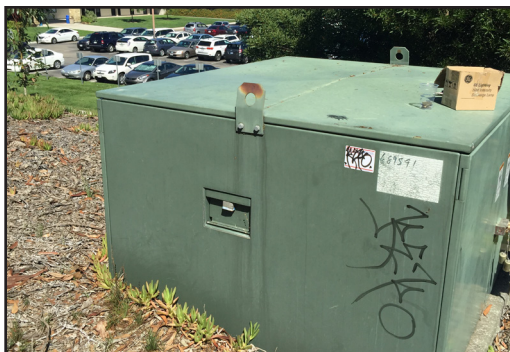
15kV Selector Switch
