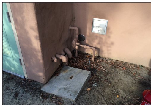
Building 200 - Gas supply into building with gas pressure regulator along building exterior.
