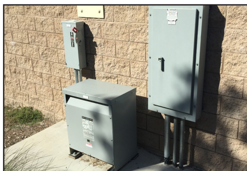
480-120/208V Transformer and 120/208V Panel Board
