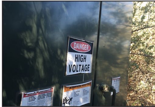
Liquid Filled Padmount Transformer
