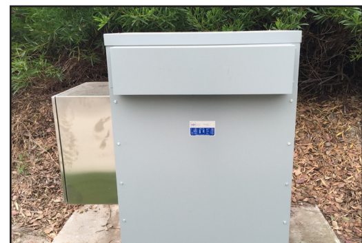
Main 150kVA 4.16kV-120/208V Transformer
