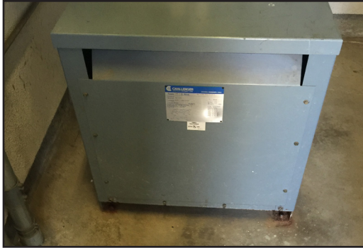
Building 900 - Typical 480-120/208V transformer
