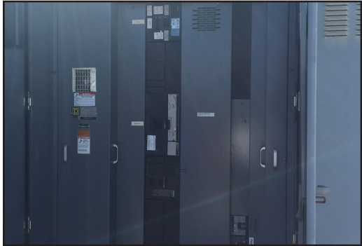
Main Distribution Board
