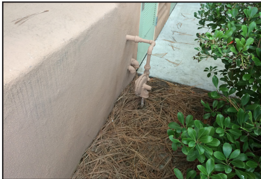
Building 600 - Gas supply into building with gas pressure regulator along building exterior.
