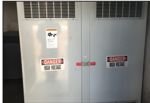
4.16kV-277/480V Dry-type Transformer
