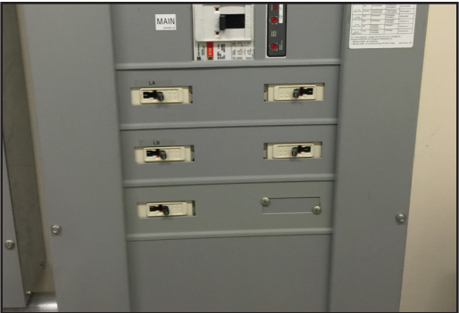
Main Distribution Board 120/208
