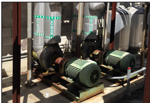
Condenser Water Pumps
