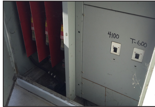
Main 4.16kV-120/208V Transformer
