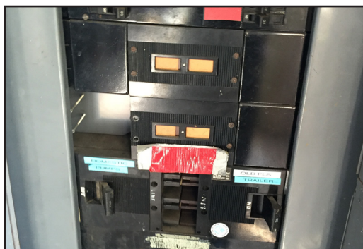
Main Distribution Board in Electrical Power House
