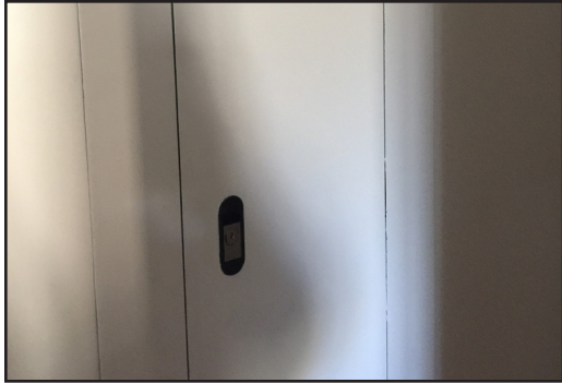
Building 1000 - 120/208V panelboard
