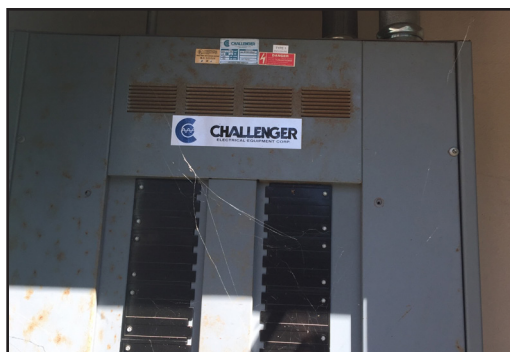
Building 100 - Main Distribution board
