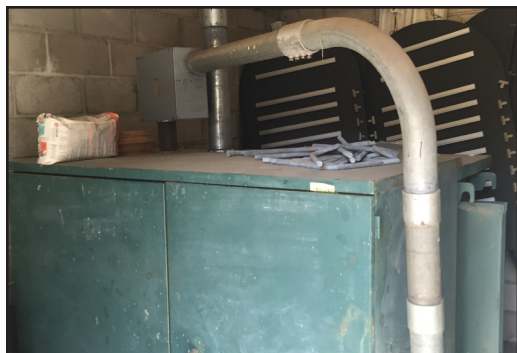
Main 4.16kV-120/208V Transformer
