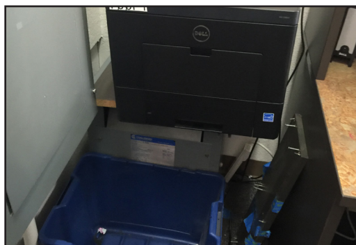
Building 700 - 480-120/208V transformer
