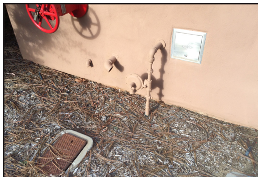
Building 100 - Gas supply into building with gas pressure regulator along building exterior.
