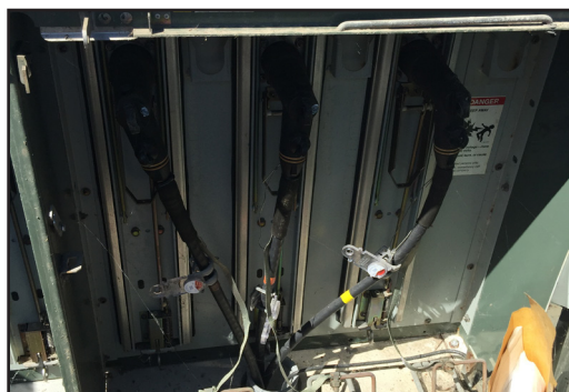
15kV Selector Switch
