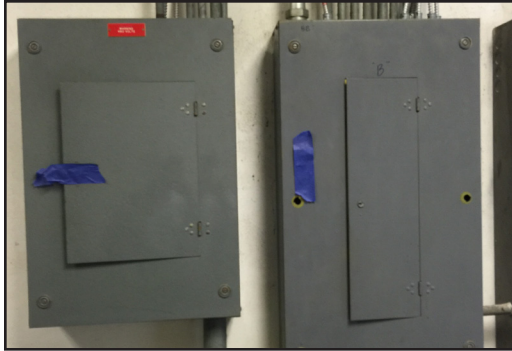
Building 3500 - 5kV Switch
