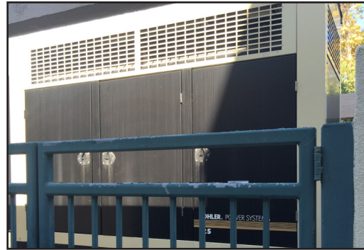
Generator Serving Existing Data Center
