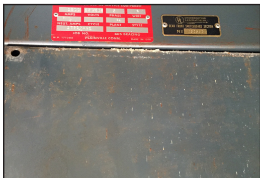
Main Distribution Board
