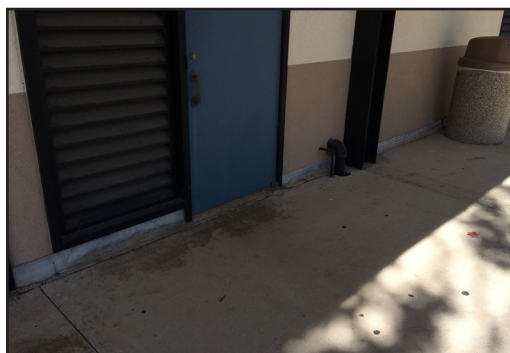
Building 4800 - Low pressure gas into building.
