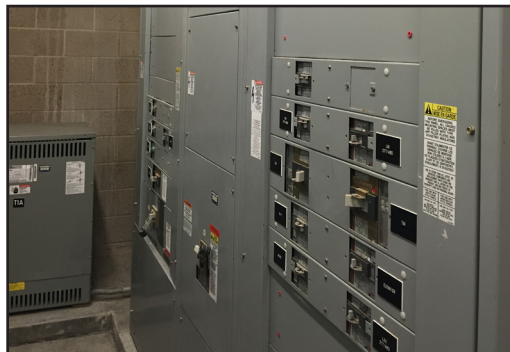
Main 277/480V Switchboard
