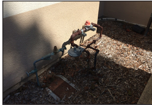
Building 5200 - Low pressure gas into building with shut-off on rise.
