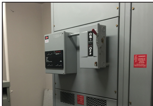
Main 1600A 120/208V Switchboard
