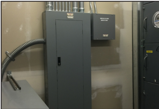
Building 900 - Typical panelboard
