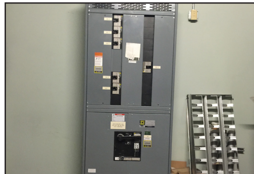
Main Distribution Board
