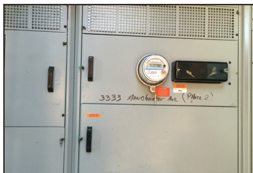
Building 500 - Main distribution board with SDG&E meter
