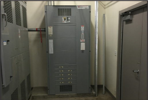
Main Equipment Room
