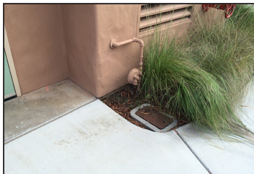
Building 800 - Gas supply into building with gas pressure regulator along building exterior.
