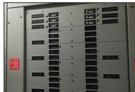
Main 1600A 120/208V Switchboard
