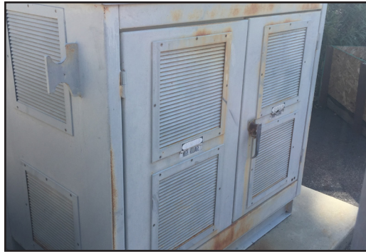
Main 4.16kV-120/208V Transformer
