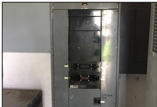
Main 120/208V Distribution Board
