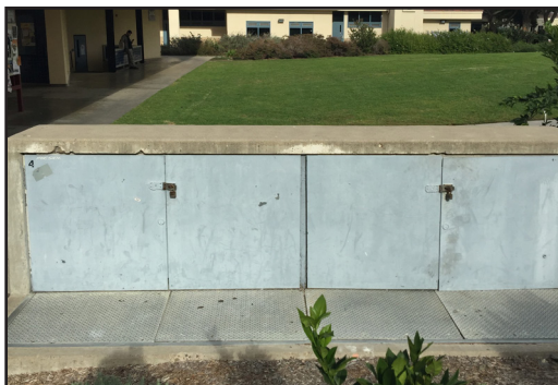
Main MV Vault
