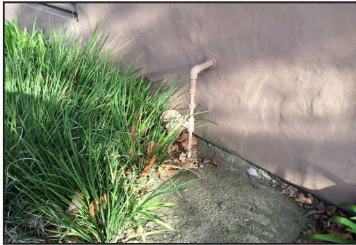
Building 400 - Gas supply into building with gas pressure regulator along building exterior.
