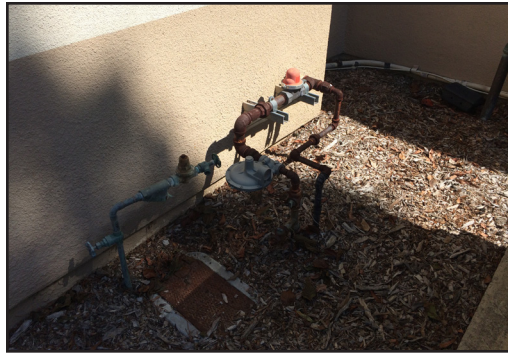
Building 4400 - Above grade gas pressure regulator along building exterior on the south side of the bldg.
