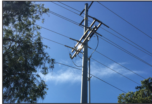
Overhead SDG&E service to campus from Barnard Drive
