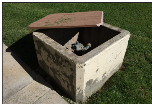
Building 1000 - Gas Pressure regulator inside concrete vault.
