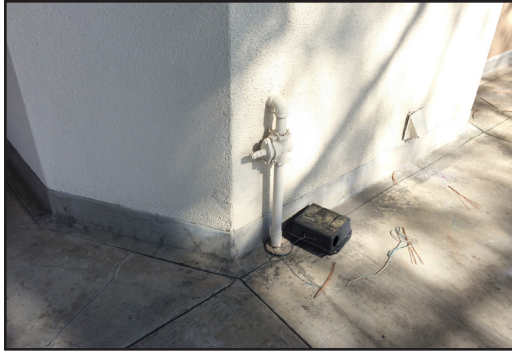
Building 2000 - low pressure gas into building with shut-off on rise.
