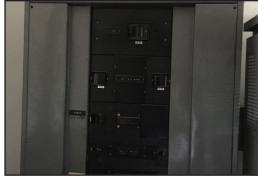
Main 277/480V Switchboard
