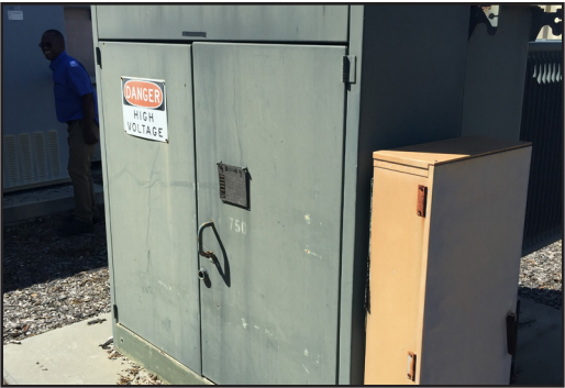
Abandoned Padmount Transformer
