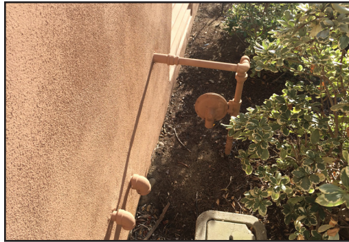
Building 500 - Gas supply into building with gas pressure regulator along building exterior.
