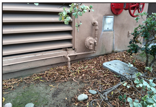
Building 300 - Gas supply into building with gas pressure regulator along building exterior.
