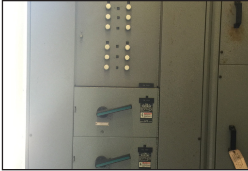
Building 600 - Main distribution board
