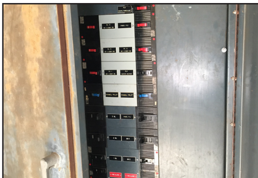
Main Distribution Board
