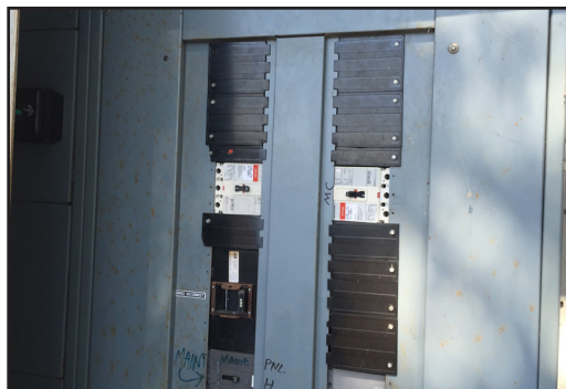
Building 700 - Main distribution board with SDG&E meter
