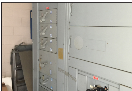
Main 1000A, 120/208V Distribution Board
