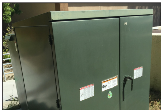
750kVA, 4.16kV-277/480V Padmount transformer
