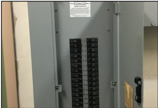
Building 900 - Typical panelboard
