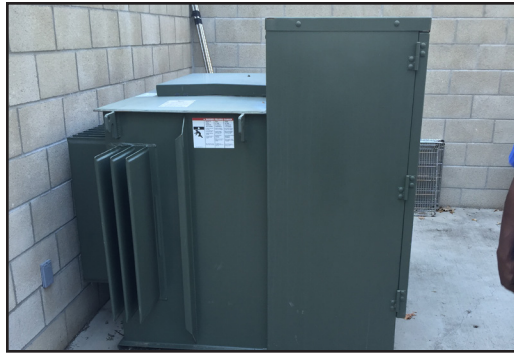
4.16kV-277/480V Padmount Transformer
