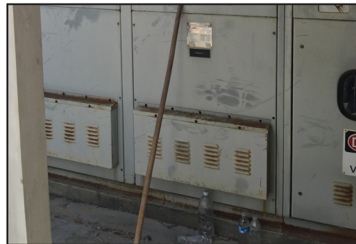
Main 277/480V Switchboard
