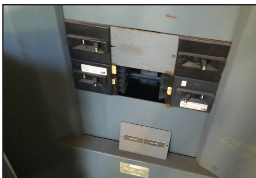
Main Distribution Board
