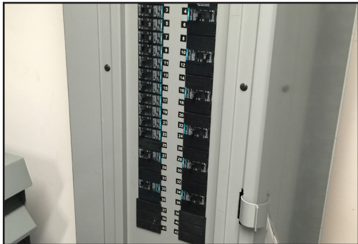
Building 1000 - 277/480V panelboard
