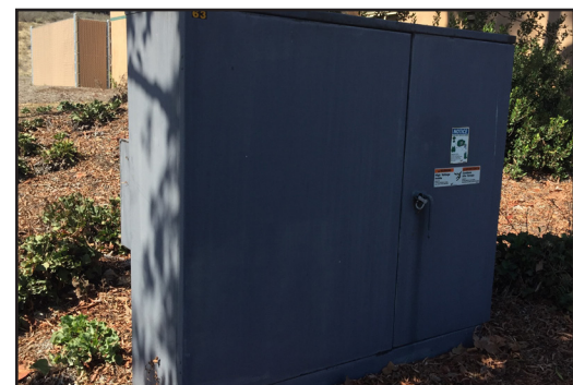
Building 700 - SDG&E pad mount transformer
