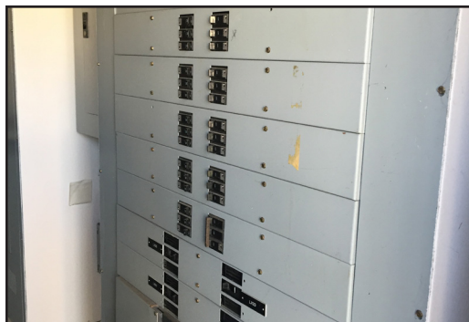
Main 1600A 120/208V Switchboard
