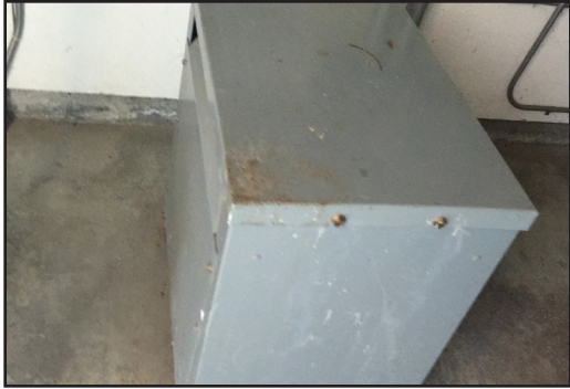
Building 600 - Typical panelboard
