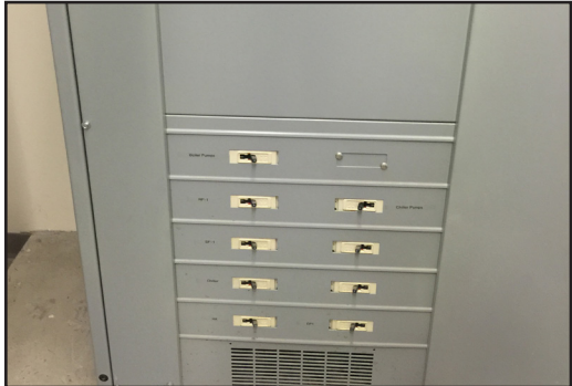
Main Distribution Board 277/480
