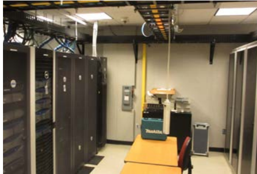
Oceanside Data Center
