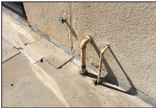
Typical rusting at natural gas line connections to buildings
