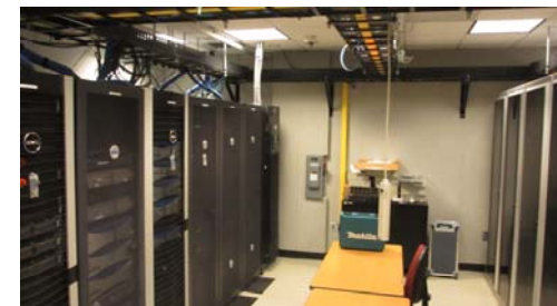
Figure 2 – Data Center (primary) Room 1264 at Oceanside campus.
