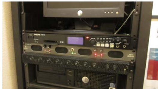
Figure 28 – Existing Boardroom equipment rack.
