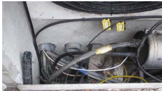
Figure 10 – Inside external vault.
