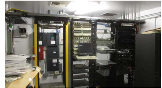
Figure 11 – Telecom room at CLC campus.
