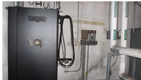
Figure 1 – Example of Communications equipment located in mechanical spaces.
