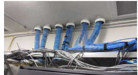
Figure 12 – Incoming services at San Elijo campus Data Center.
