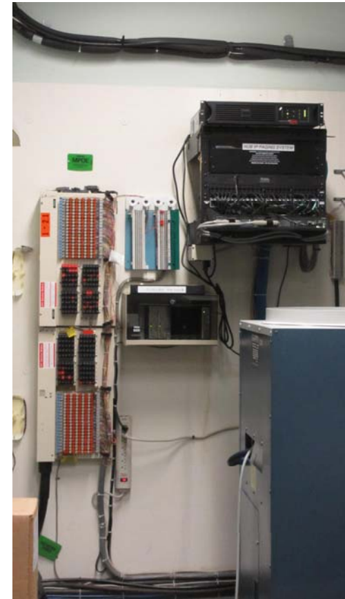
Figure 1 – Main Point of Entry (MPOE) for Oceanside service providers.
