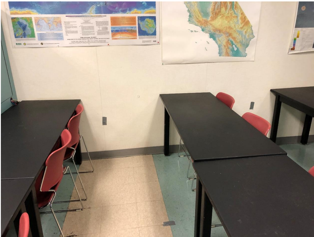
Photo 4 – Building 400 / Room 406, Fiberboard at North Wall.
