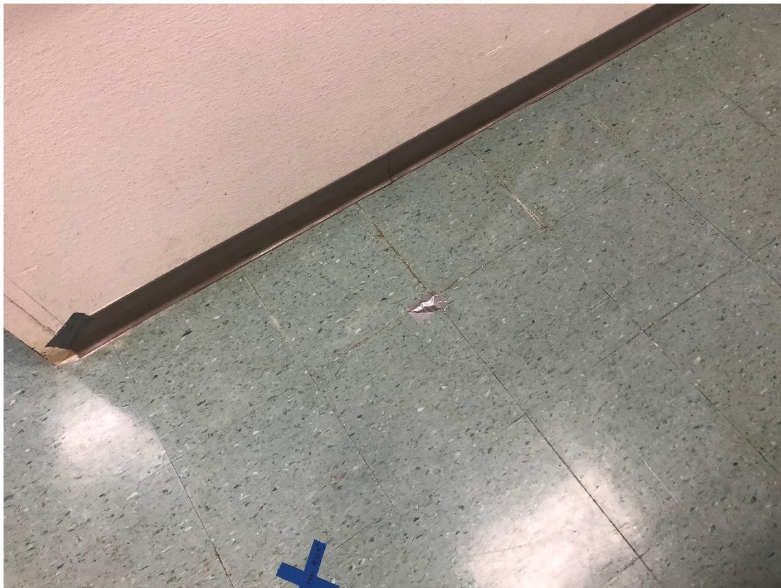
Photo 6 – Building 400 / Room 406, 12" X 12" Vinyl Floor Tile (Green Speck) w/ Mastic & 4" Vinyl Cove Base (Grey) w/ Adhesive
