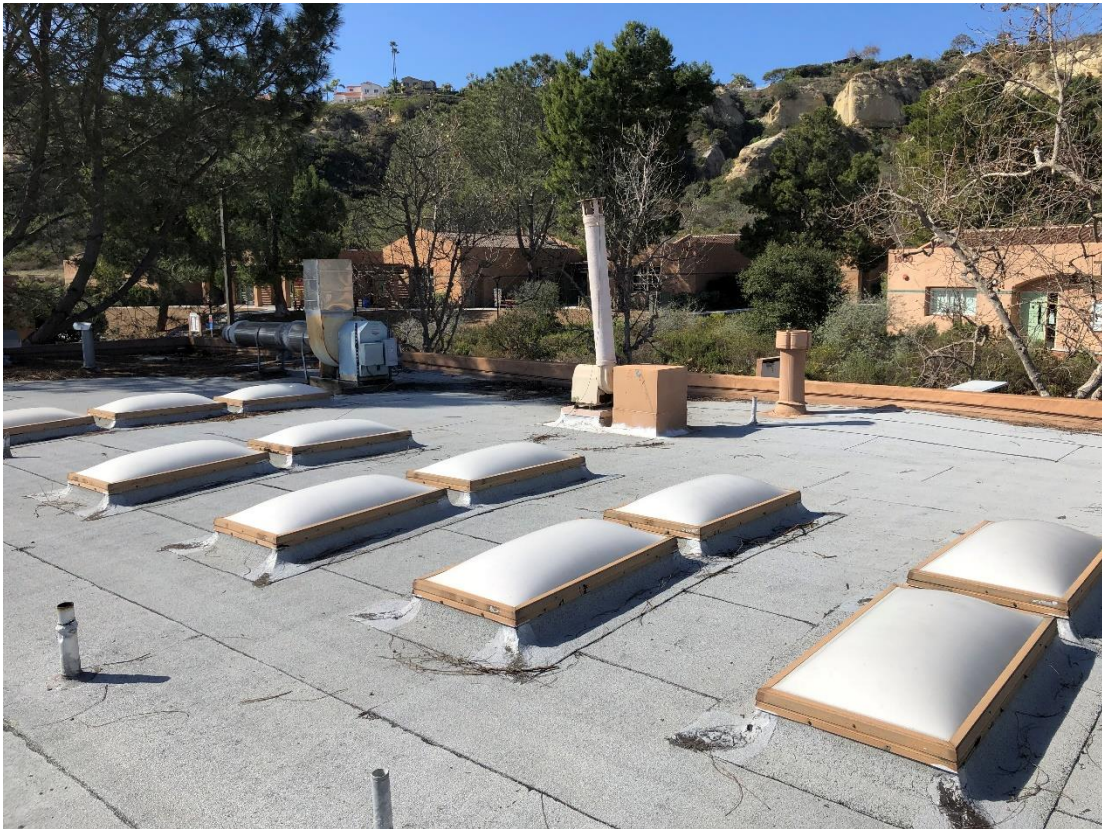
Photo 16 – Building 400 / Exterior Main Roof, Penetration Mastic at East Skylight.
