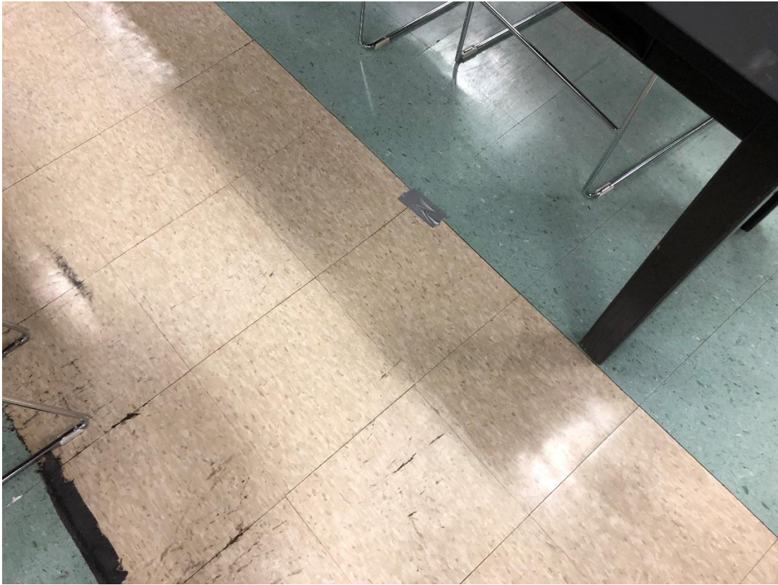
Photo 7 – Building 400 / Room 406, 12" X 12" Vinyl Floor Tile (Beige Speck) w/ Mastic.
