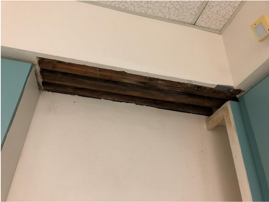
Photo 3 – Building 400 / Room 406, Drywall, Tape & Joint Compound at SE Soffit.
