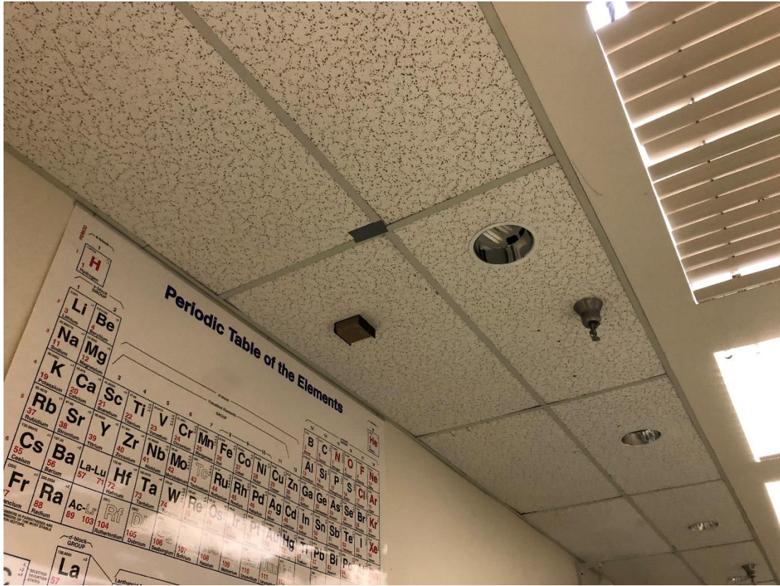
Photo 5 – Building 400 / Room 402, 2' x 4' Rough Fissured Ceiling Tile.
